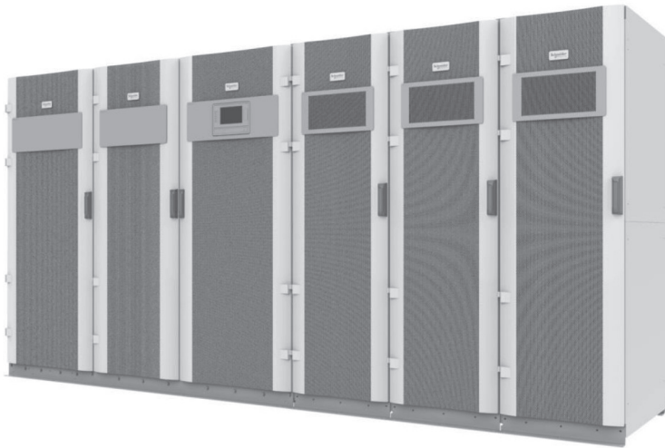
Figure 3 An example of a UPS with li-ion batteries is the Galaxy VX from Schneider Electric
